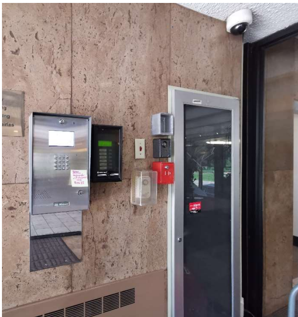
Access Panel and Fire Alarm Panel
