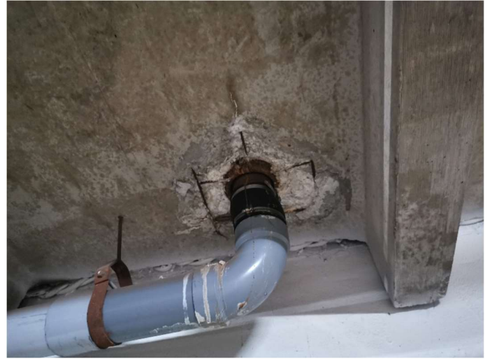
Leak in Parkade from Hot Tub
