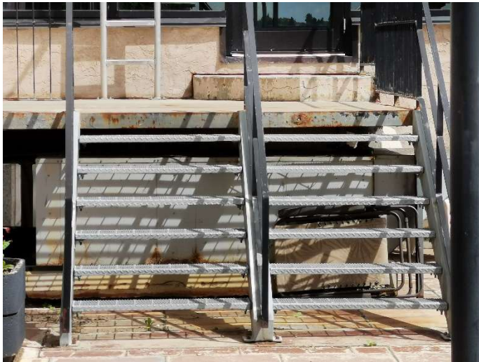
View of Courtyard – Metal Stairs and Makeup Air Unit (Smoke Removal)
