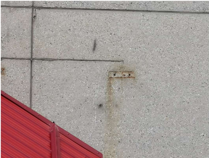
Views of Cracks in Building Envelope (East)
