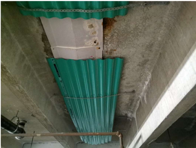
Parkade: View of Past Repairs
