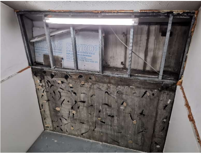
View of Leak in Roof of Pool Facility
